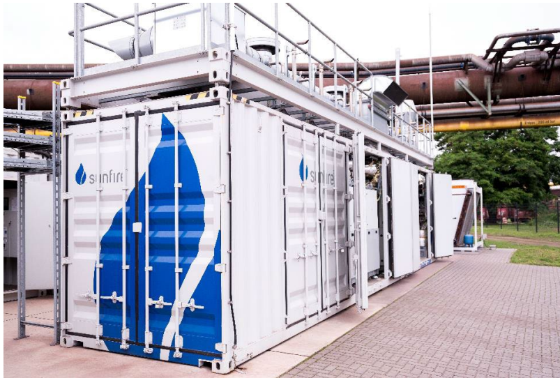
GrInHy2.0 high-temperature electrolyzer at Salzgitter's steel works (© Salzgitter AG)
