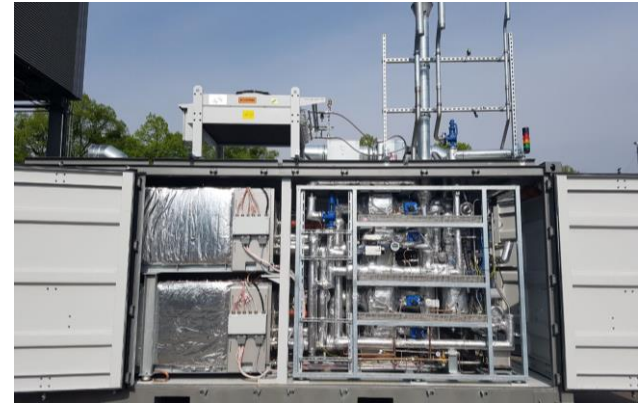
150 kW SOEC module in Salzgitter, Germany
