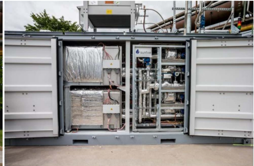
Fig. 2. Container of the Reversible Solid Oxid Cells (1440 rSOCs in 6 modules)
