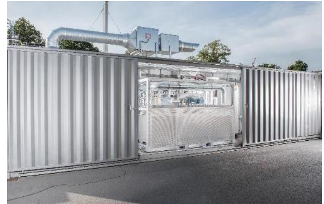
Commissioning at sunfire site, Germany
