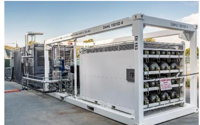
RSOC installation at Navy base in Los Angeles, USA
